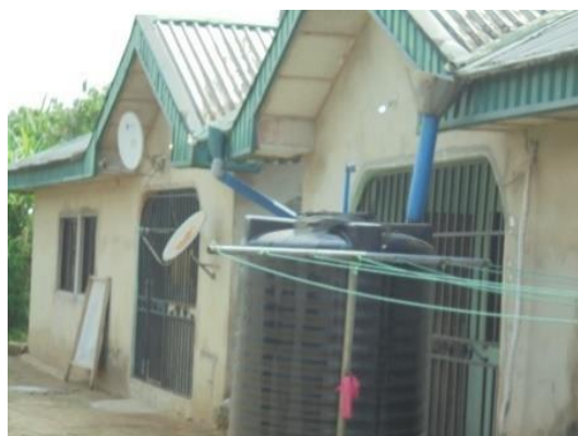
Plate 4.15: Rainwater collection system in Nedugo community
