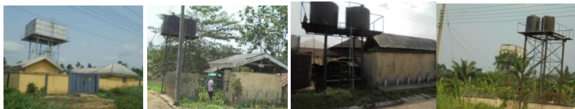
Plate 4.14: From Left to Right - Non-functional water facility at Agbia, Okotiana, Nyambiri and Zarama-Epie communities
