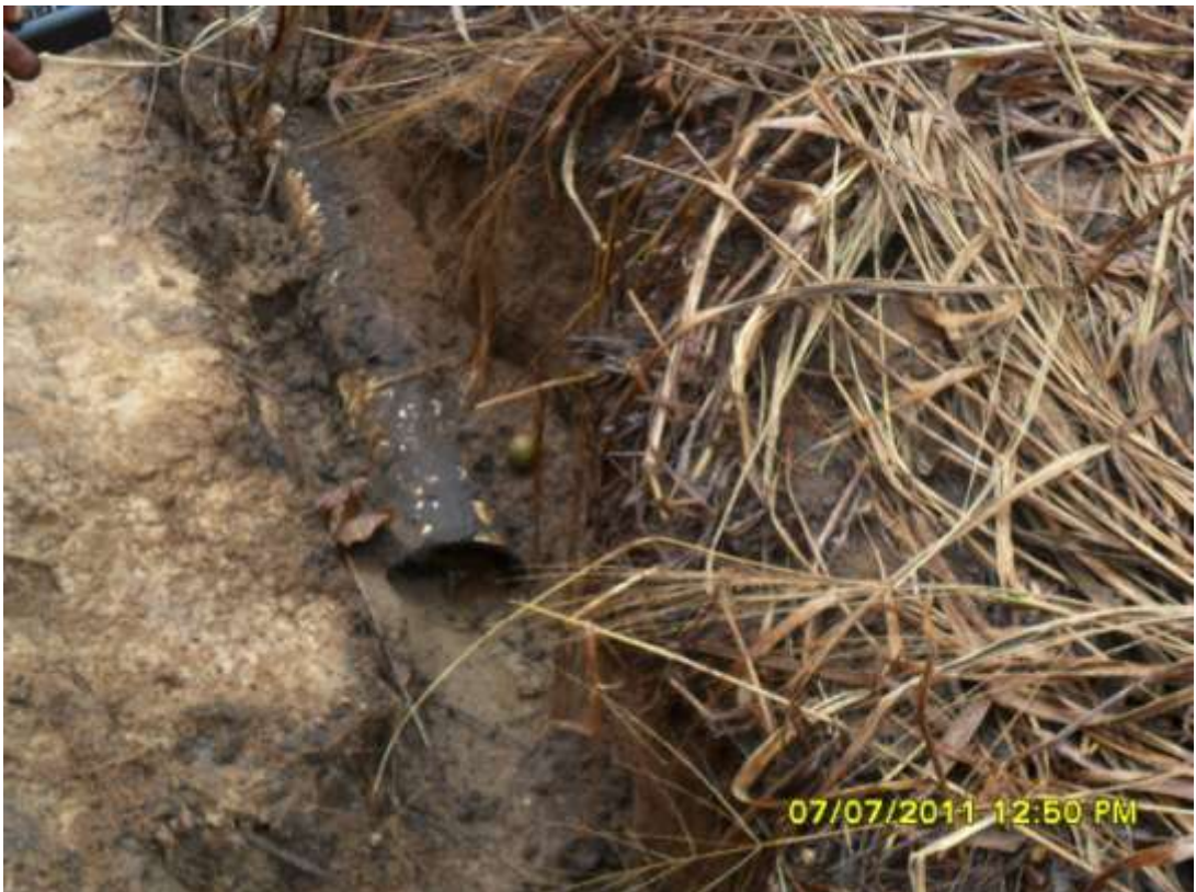
Close-up: Cut section on Ubie Well4S flowline at Ubie. Picture taken during Joint Investigation of 7 th July, 2011
