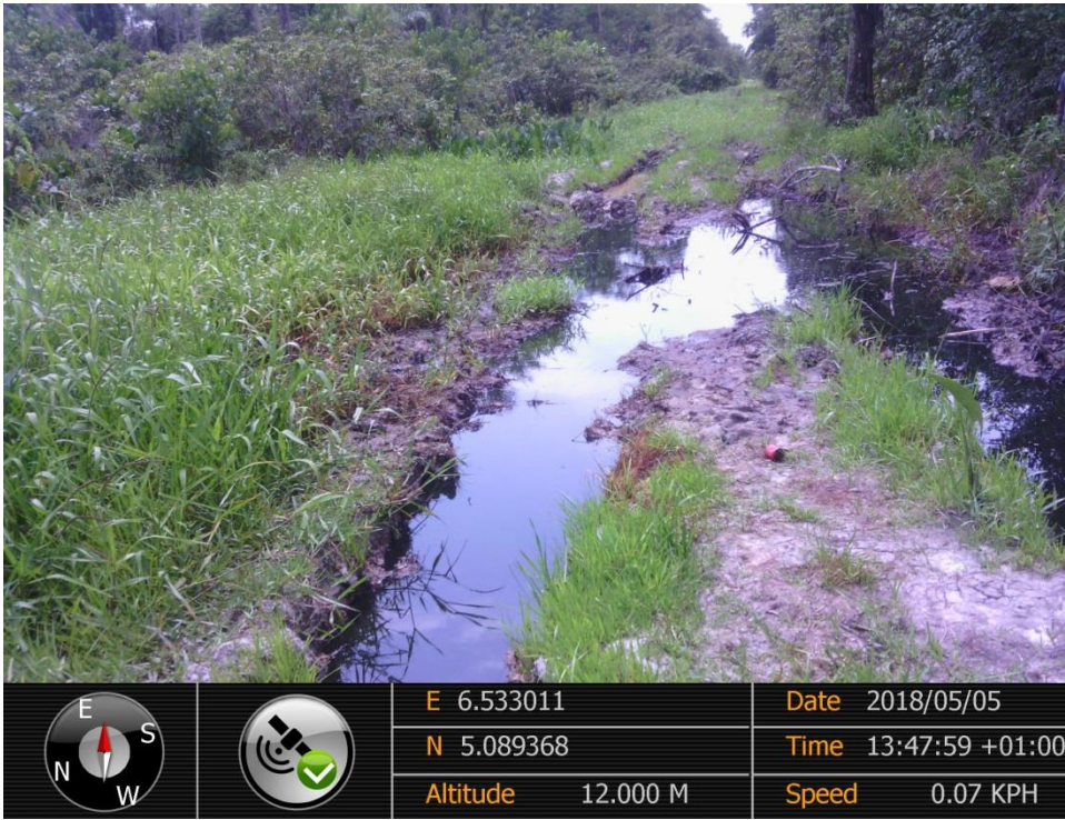
Overview: Part of spill impact on 14" Okordia – Rumuekpe Pipeline at Ukpeliède. Picture was taken during Joint Investigation of 5 th May 2018.
