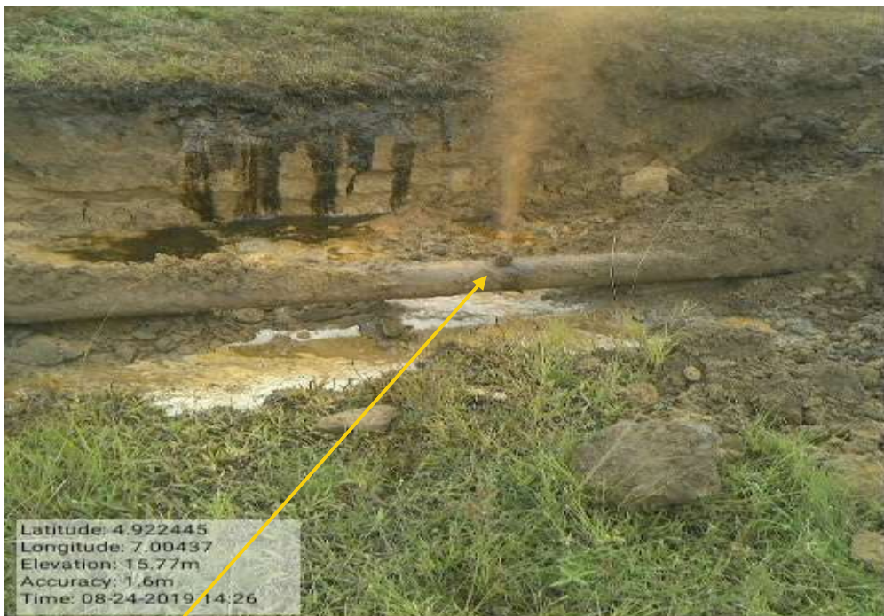
Close-up: Illegal fitting on 8"Umuechem – Nkpoku Deliveryline at Rukpokwu. Picture was taken during Joint Investigation of 24 th August 2019.
