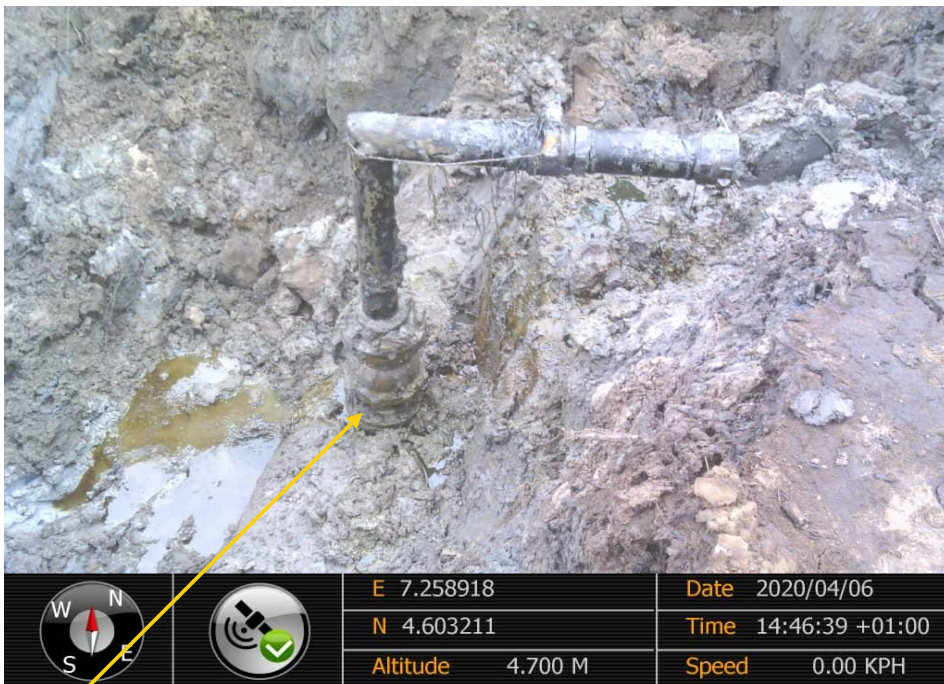
Close-up: 6" crude oil theft valve installed at 12 o'clock position on 28" Bomu Bonny Pipeline at Bodo. Picture was taken during Joint Investigation of 6 th April 2020.
