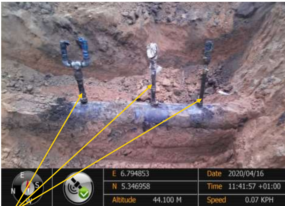
Close-up: 3nos of crude oil theft points at 12 o'clock position on 18" Assa- Rumuekpe Pipeline at Ochia. Picture was taken during Joint Investigation of 16 th April 2020.
