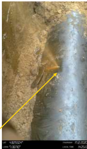
Close-up 1: Rectangular hole of 12mmx15mm created 10 o'clock position on 36inch Nkpoku Ogale Pipeline at Agbonchia. Picture was taken during Joint Investigation on 21st Dec 2020.
