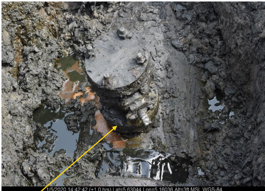
Close-up: Illegal fitting on 20'' Trans Escravos Pipeline at Ugboegugun. Picture was taken during Joint Investigation of 5 th January 2020.
