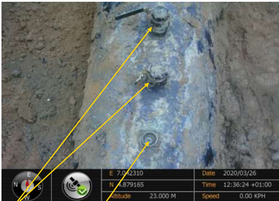
Close-up: 2nos 2" ball valves and 1 no 1" nipple installed at 12 o'clock position on 28" Nkpoku Bomu Pipeline at Rumuewhara. Picture was taken during Joint Investigation of 26 th March 2020.
