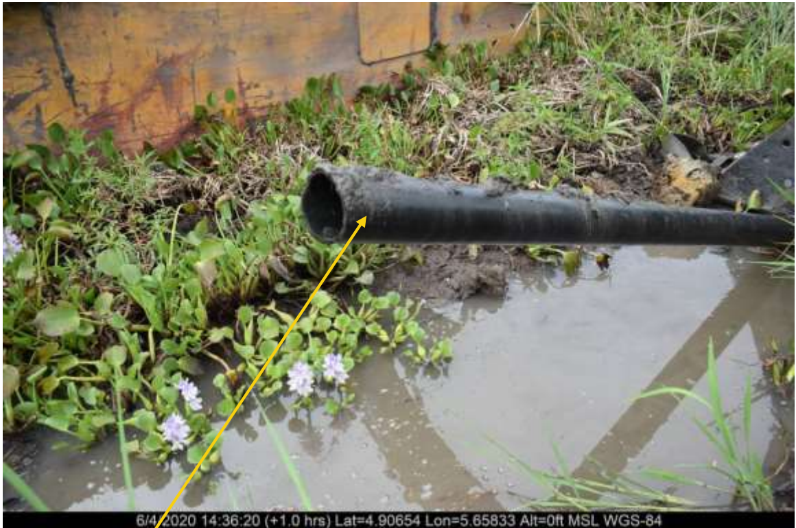
Close-up 2: 2.1km missing flowline on 4" Kanbo well 5 Lima flowline at Tunu. Picture was taken during Joint Investigation 4th June 2020.
