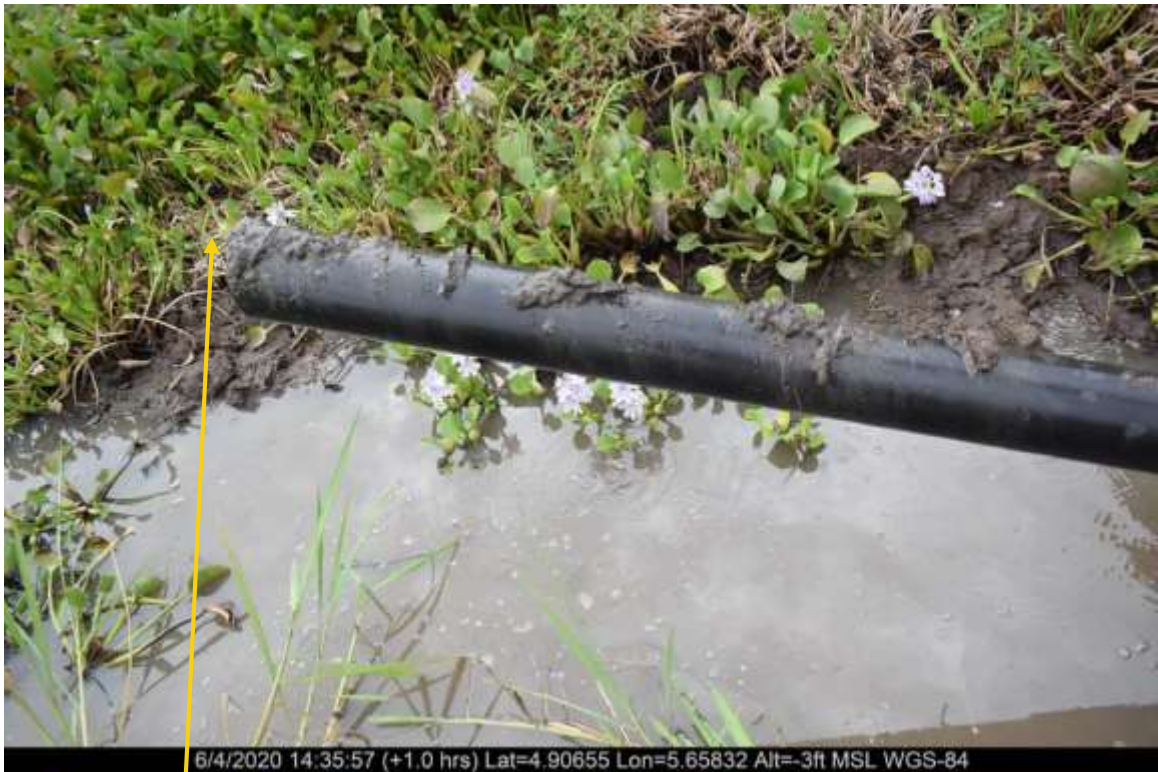
Close-up 1: 2.1km missing flowline on 4" Kanbo well 5 Lima flowline at Tunu. Picture was taken during Joint Investigation 4th June 2020.
