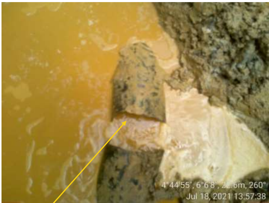
Close-up: Rupture by suspected external impact on 10" Diebu Creek Nun River Deliveryline at Eniwari/Onyeoma. Picture was taken during Joint Investigation of 18 th July 2021.
