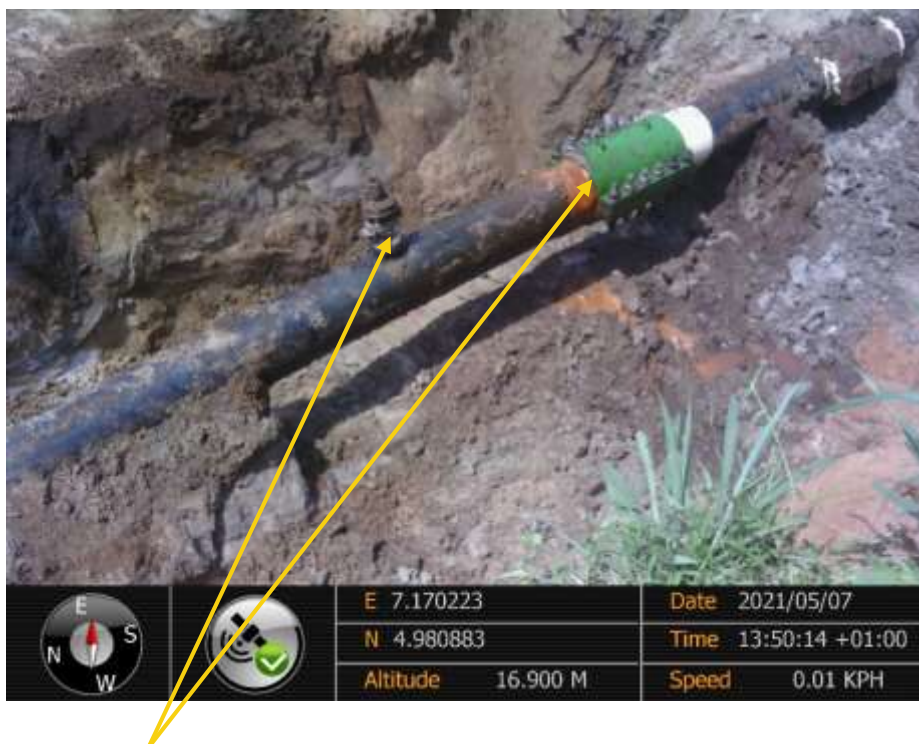
Close-up: Third Party tampering with clamp. Also 1.5m distance from the clamp is a newly installed 2inch non leaking ball valve at 12 o'clock position on 12inch Imo River 2 – Ogale Pipeline at Odagwa. Picture was taken during Joint Investigation of 7 th May 2021.
